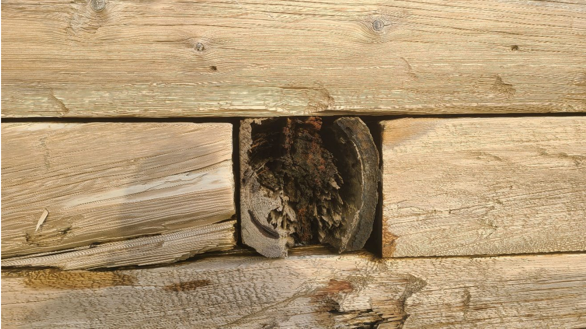
Figure 24: The end of the tie back is compromised due to rot.
