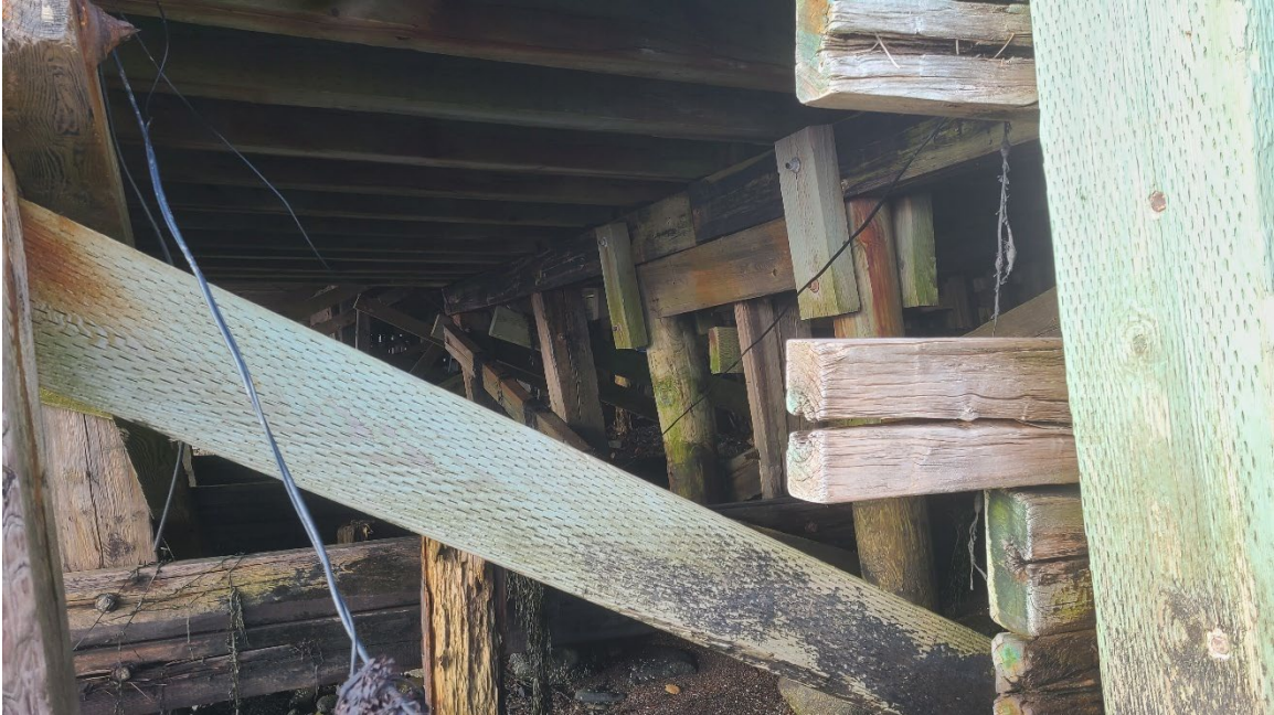
Figure 25: Leaning underside of Market Wharf deck.
