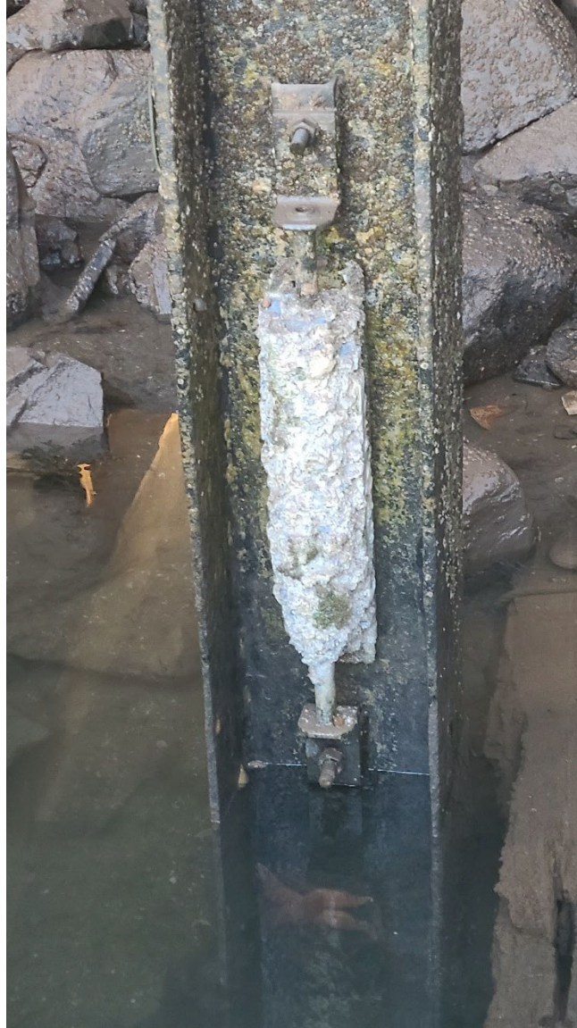
Figure 17: Structural H pile with significant hour glassing / loss of pile steel.
