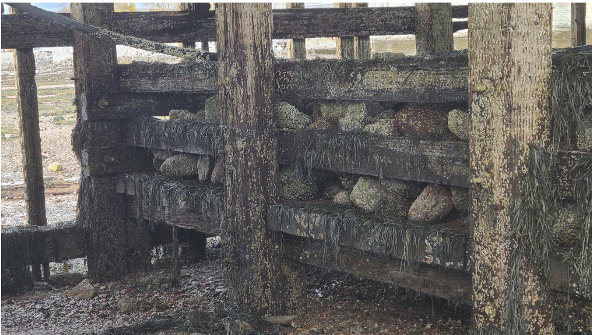
Figure 5: Line C trestle column is compromised.
