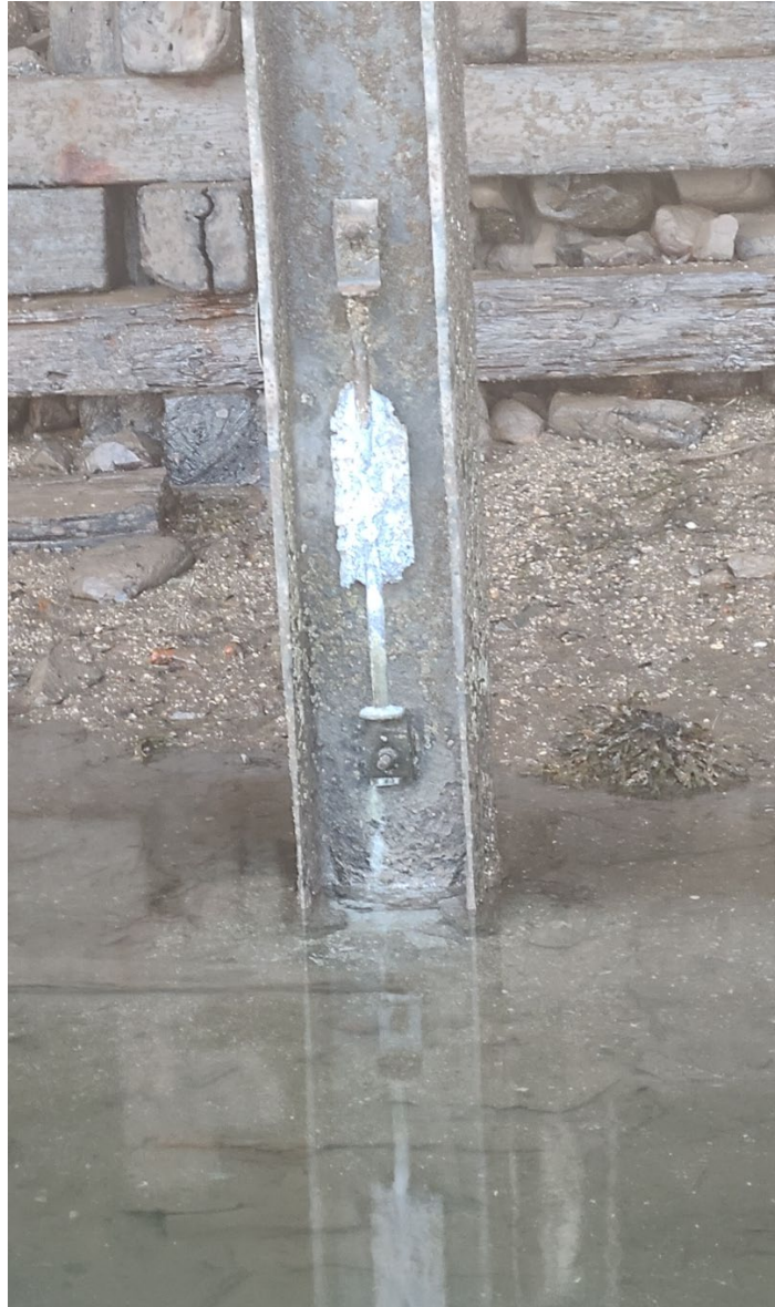
Figure 18: Structural H pile showing anode depletion and severe hour glassing / loss of pile steel.
