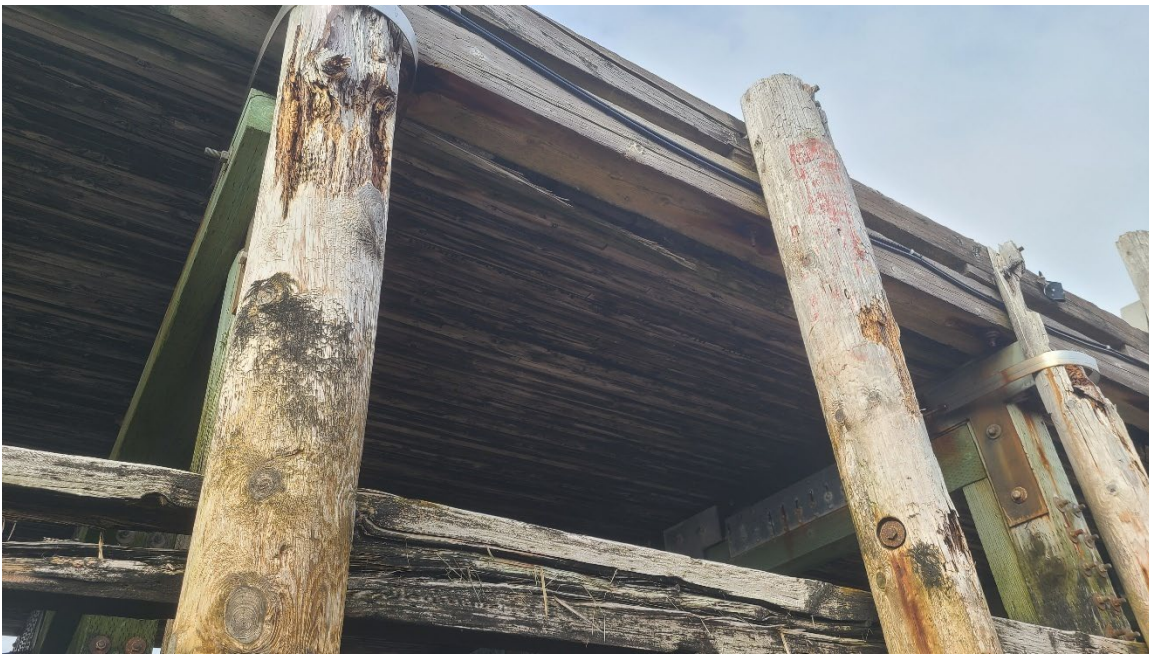
Figure 3: Between bents deck rot at edge of the wharf in numerous locations.
