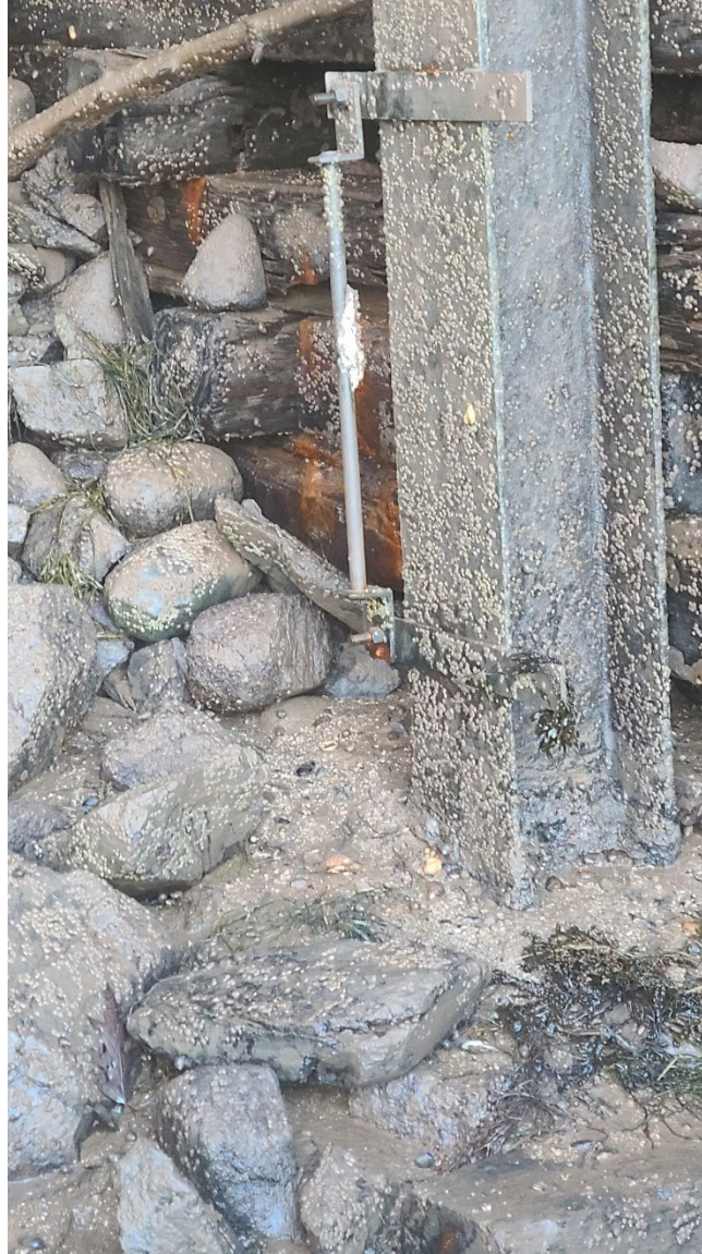
Figure 19: Sacrificial anodes in very poor condition.
