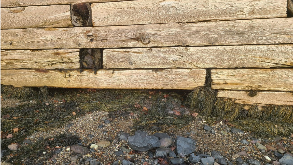
Figure 22: Void at bottom of Market Wharf (May be related to Figure 24)
