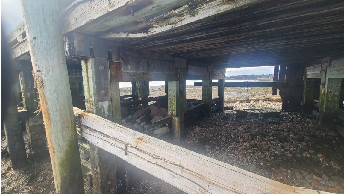
Figure 2: Collapsed Ballast Floor.
