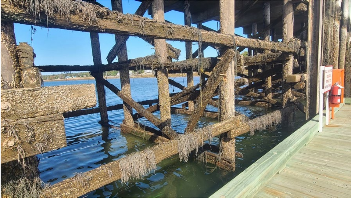
Figure 9: Walers and cross bracing are in poor condition.
