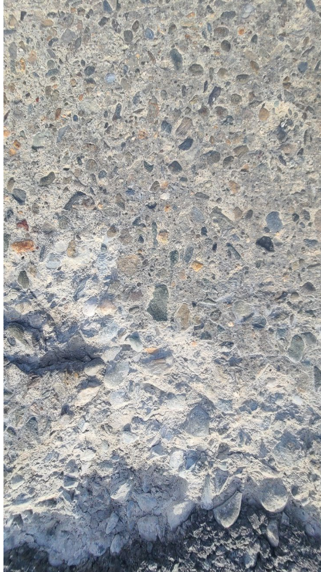
Figure 8: Alkaline Reactivity on Inner Approach Wharf concrete decking
