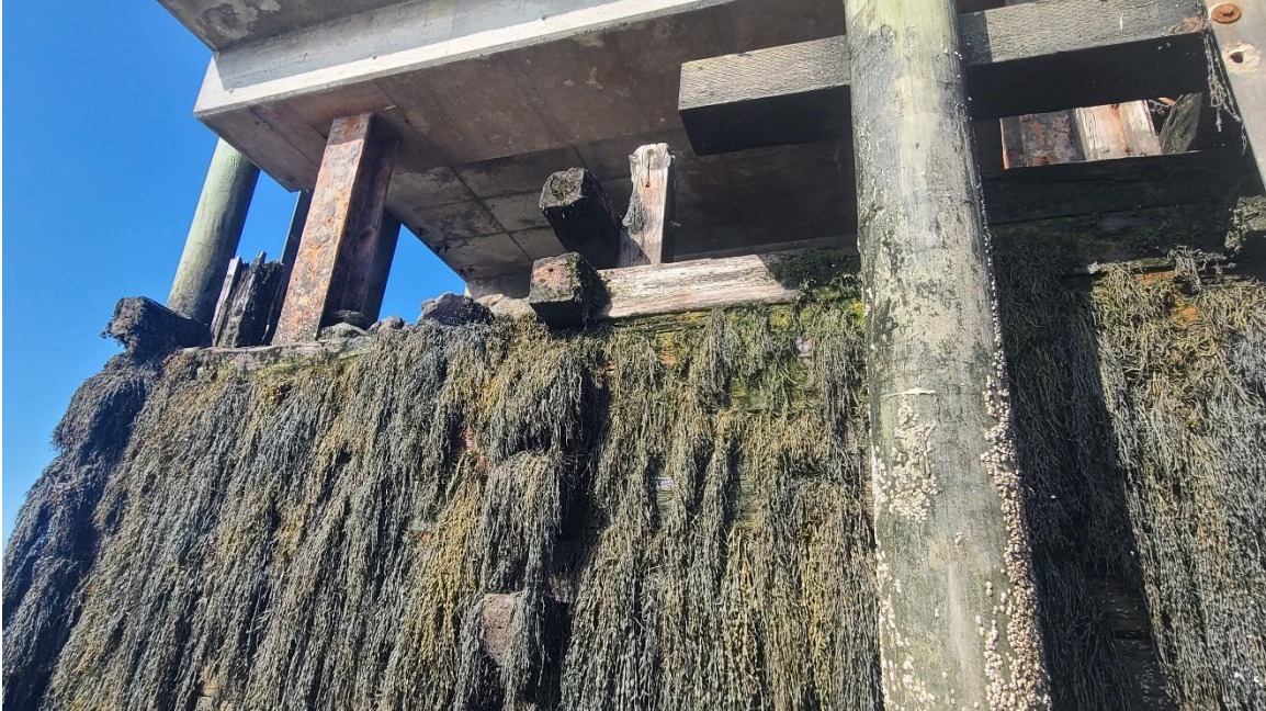
Figure 12: H Pile at Southeast Corner (Pile 22-A) with Corrosion in Splash Zone.
