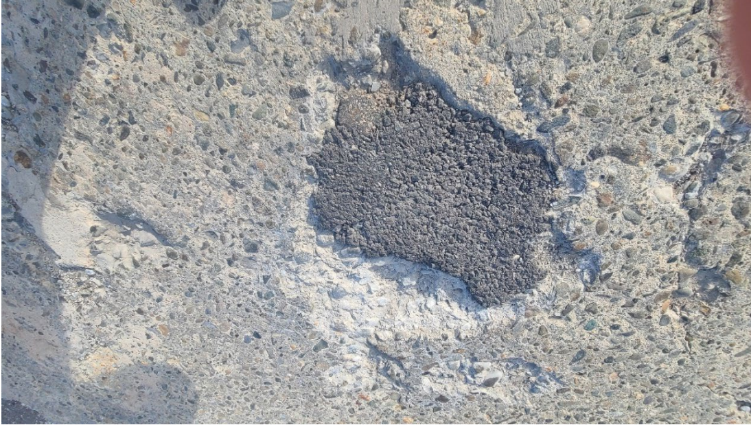
Figure 7: Inner Approach Wharf Deck Patch (200 x 450 mm) in Need of Repairs.
