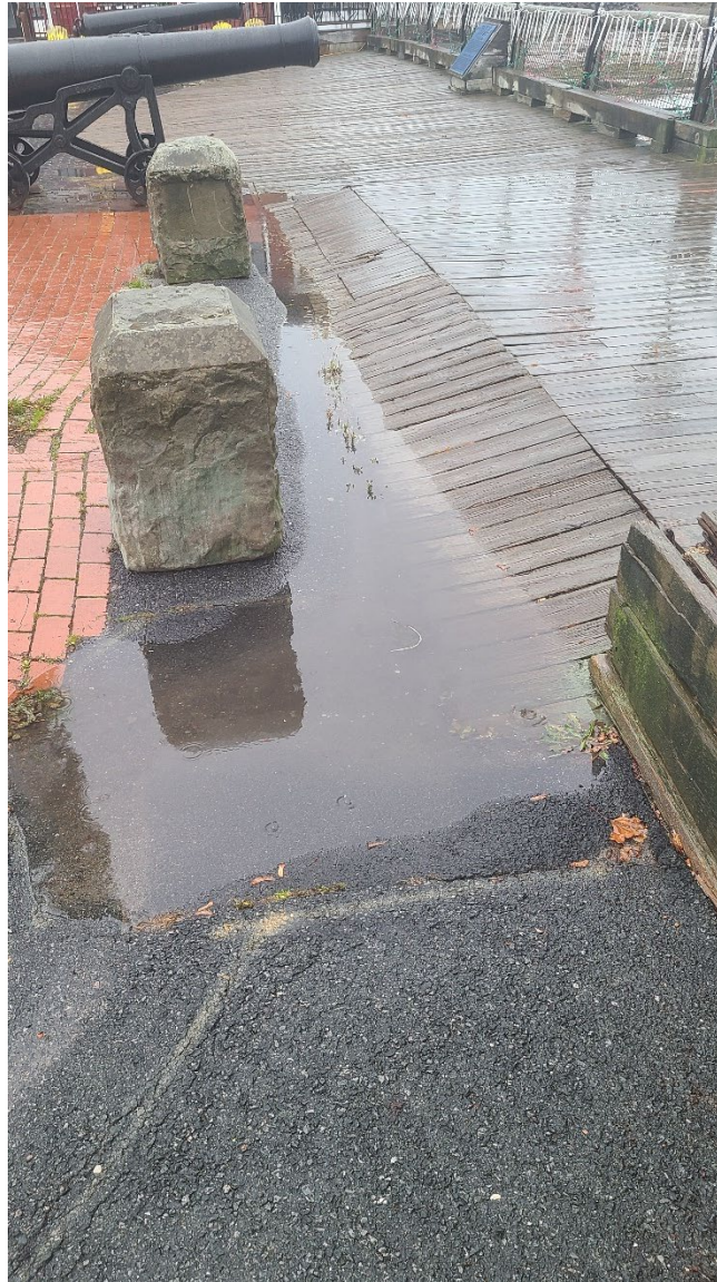
Figure 23: Subsidence behind Market Wharf crib structure.
